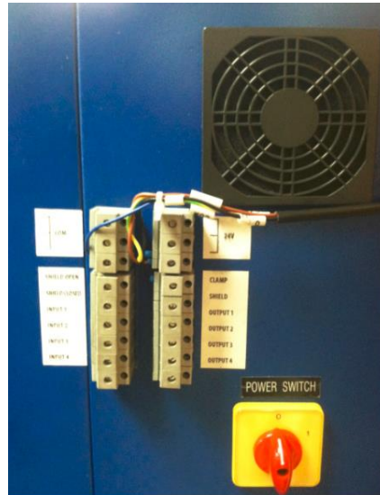
The I/ ports located at the right side of the machine
